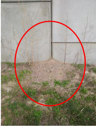
Loss of Backfill
