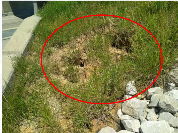
Subsidence due to loss of backfill
