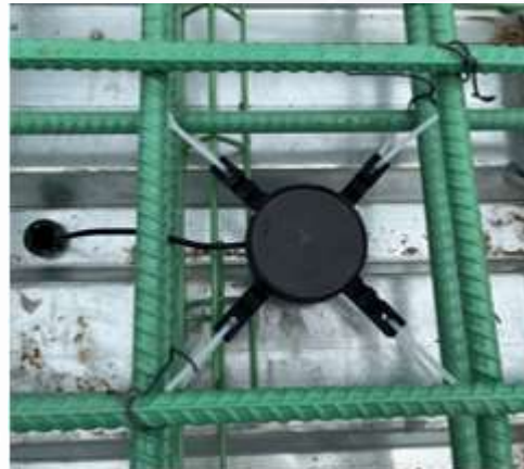
Sensor installed at Deck
